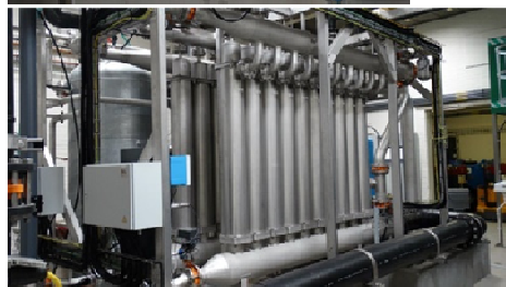
Ceramic Microfiltration In 'waste water area'
