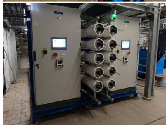
RO installation in 'Drinking water area'. At borders feed and permeate tanks. IBC tanks for chemical cleaning.
